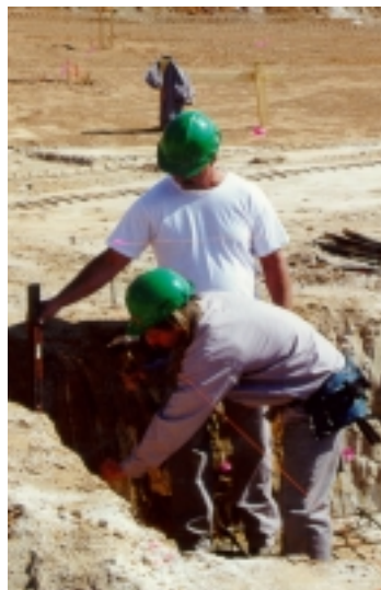
Inmates in the Inmate Construction Program work on a 208-bed dormitory addition to the NC Correctional Institution for Women in Raleigh.
